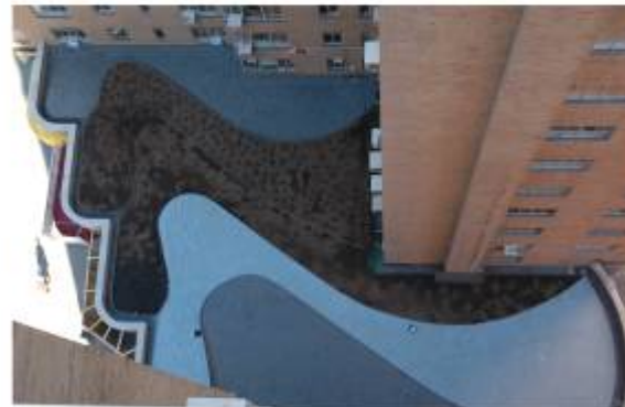
AFTER: A Green Roof is currently being planted on all lower roofs of the building.
