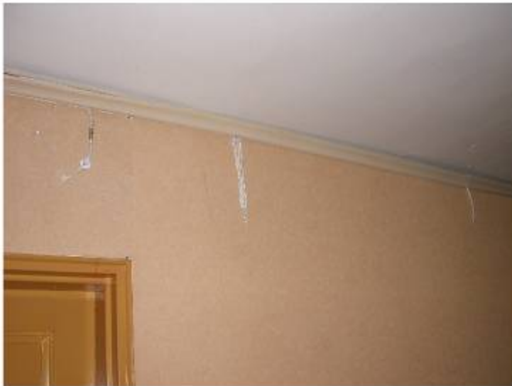
BEFORE: Typical condition.
